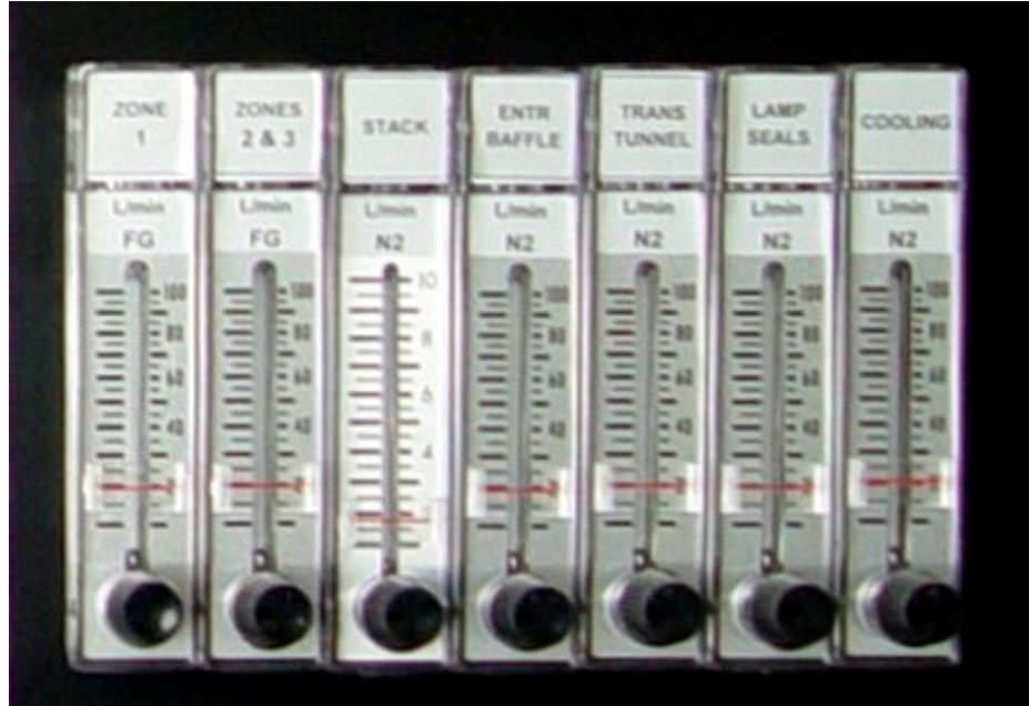
Figure 1-17 Gas Flow Control Panel
