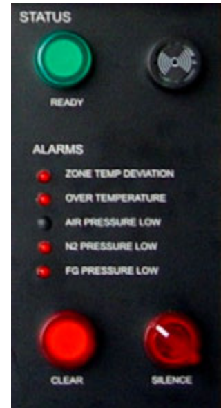
Figure 1-16 Status Panel and Alarm Controls
