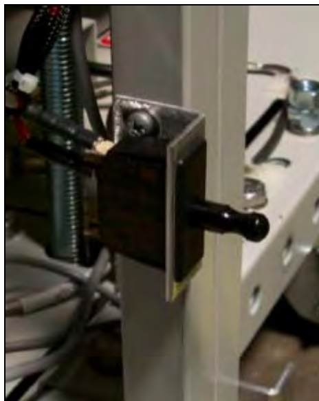
Figure 2-2: Panel Switch Installed (Override Mode Position)
