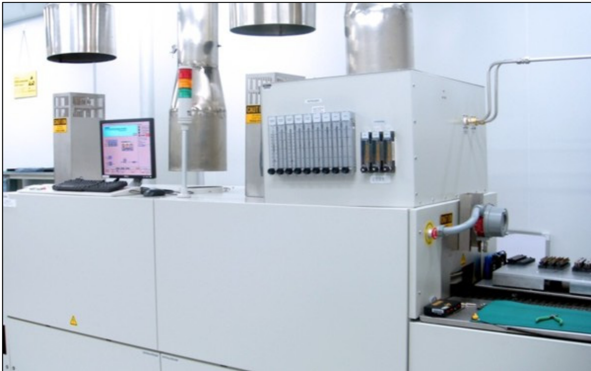
Figure 2-17 Typical Hydrogen Furnace Process Gas Exhaust Connection
