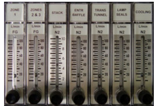
Figure 2-13 Process Gas Flowmeters
